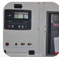
Control Panel & MCB
